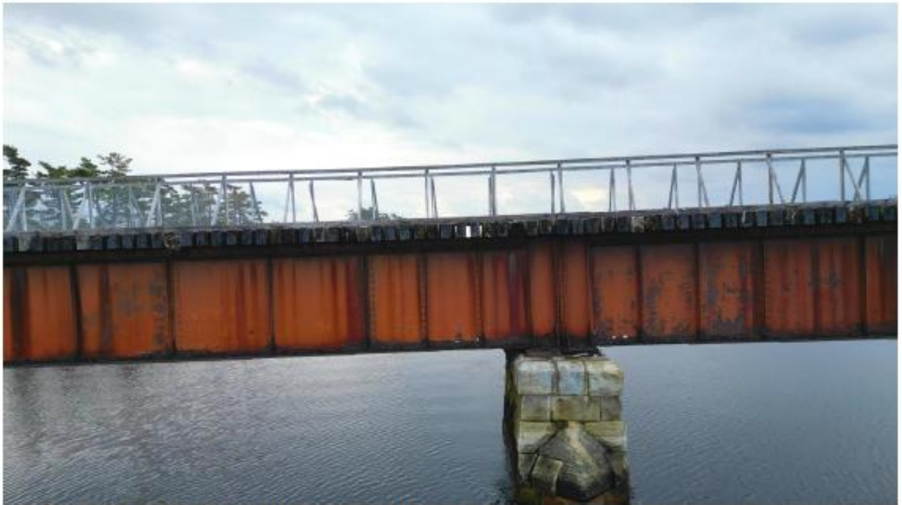
Photo 31: Areas of complete section loss in web, near east pier at north side of bridge.
