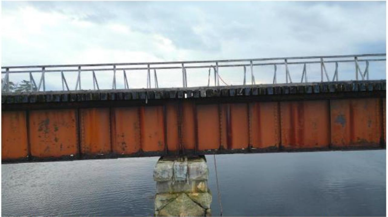
Photo 30: Areas of complete section loss in web, near west pier at north side of bridge.
