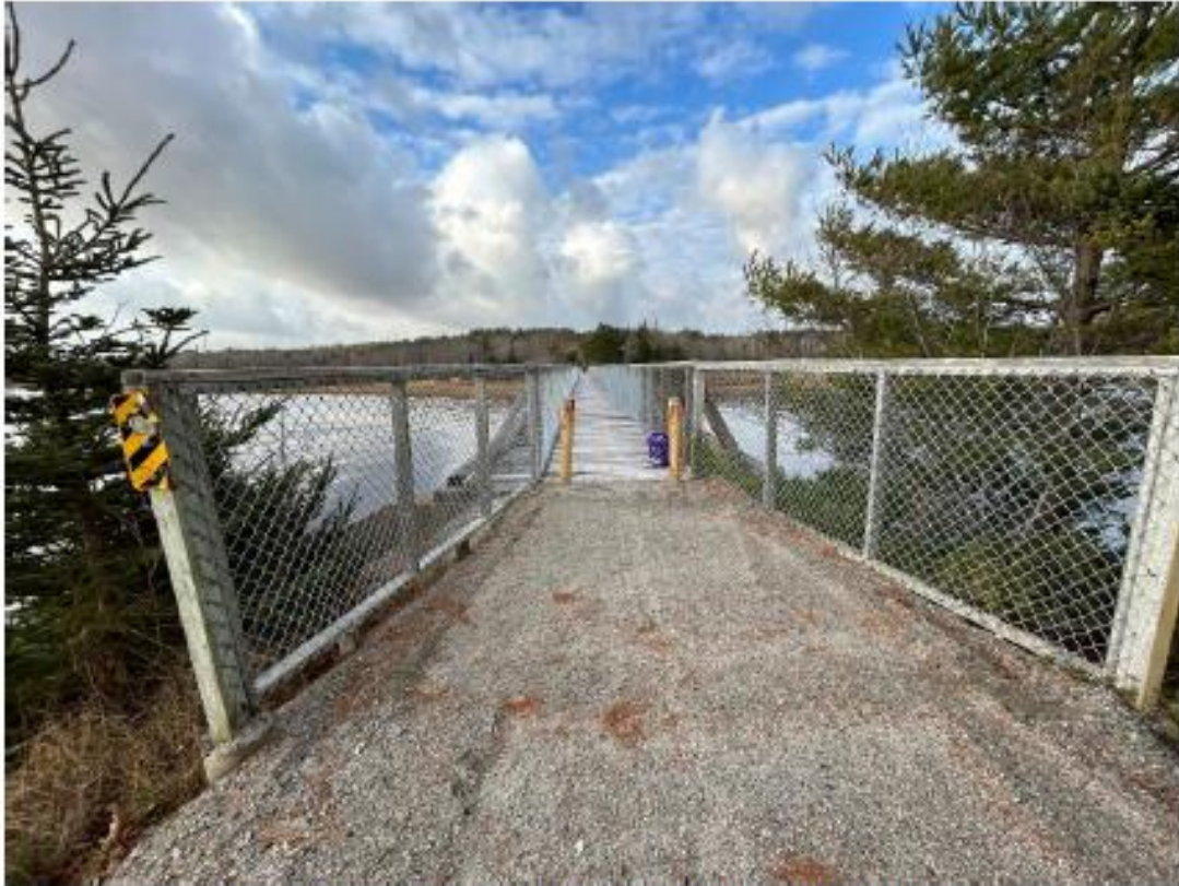
Photo 4: East approach with damaged hazard sign.
