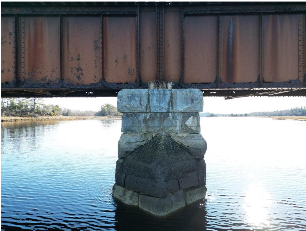
Photo 12: Typical erosion and scaling on pier nose.
