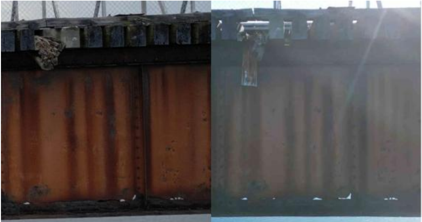
Figure 3 - North girder, Span 2 (viewed from west to east), showing condition comparison between 2023 (left) and 2025 (right). Increase in existing section loss and new areas of section loss forming.
