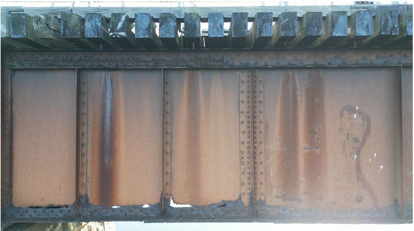
Photo 24: Severe corrosion on the north girder near the east abutment, resulting in section loss.
