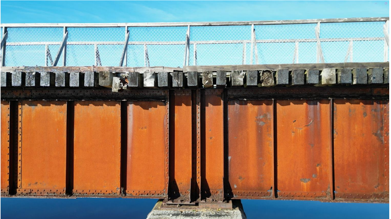
Photo 21: Severe corrosion on the south girder near the east abutment, resulting in section loss.
