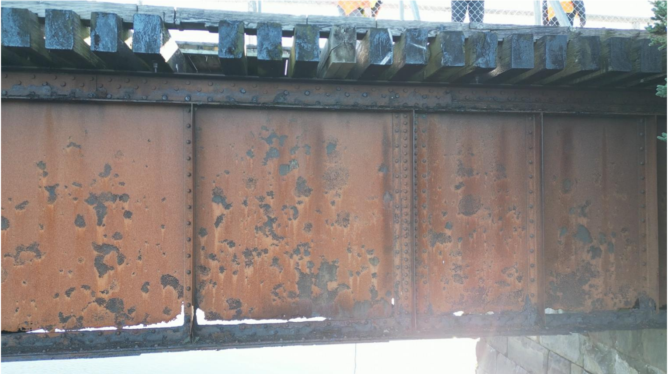
Photo 23: The most extensive corrosion on the north girder near the west abutment, resulting in severe section loss on the girder web.
