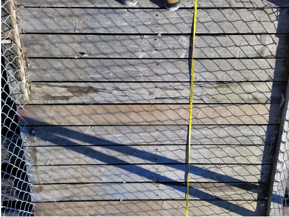
Photo 3: Typical view of timber deck planks, with several boards replaced.
