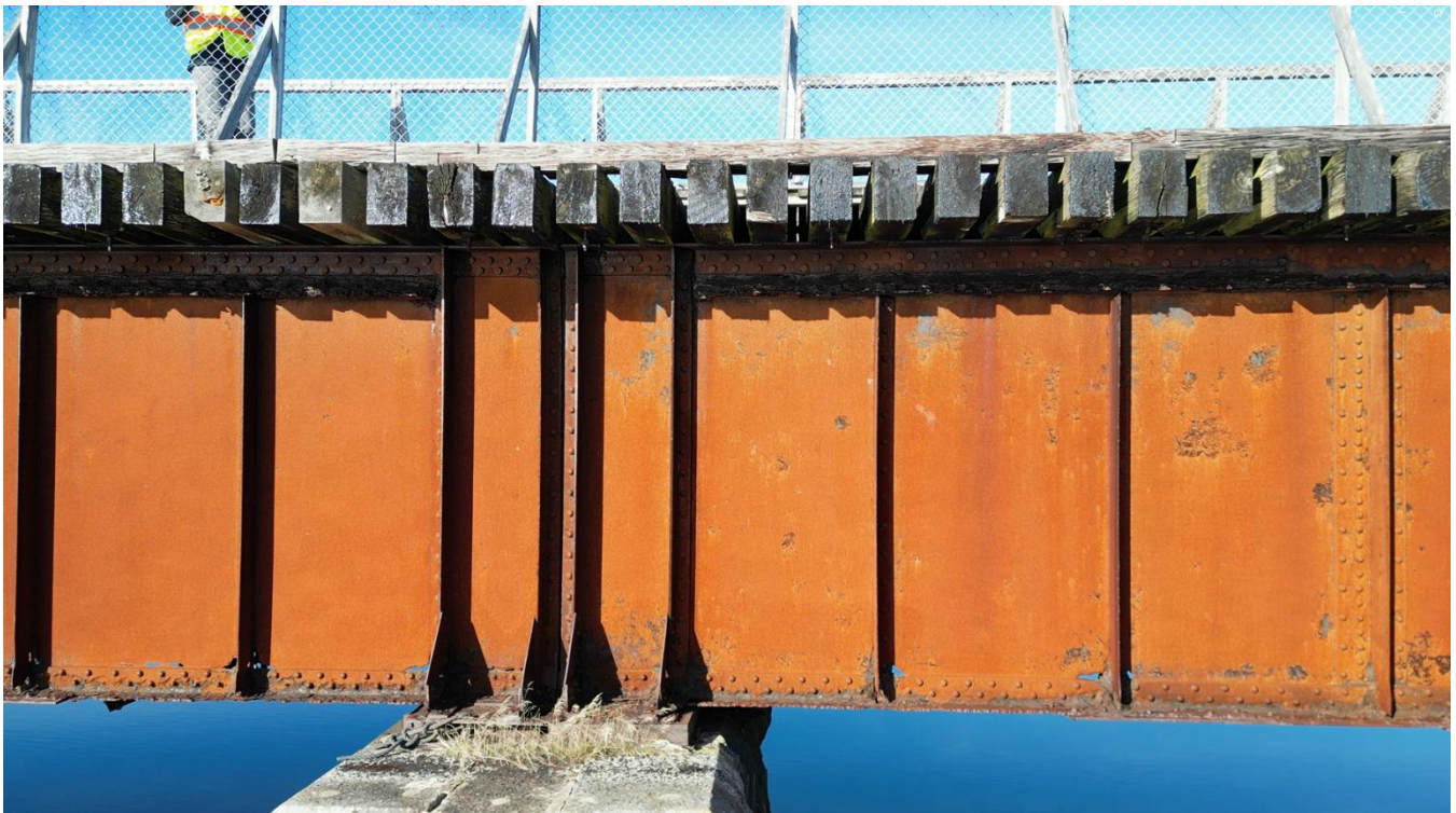
Photo 20: Severe corrosion on the south girder near the west pier, resulting in section loss.
