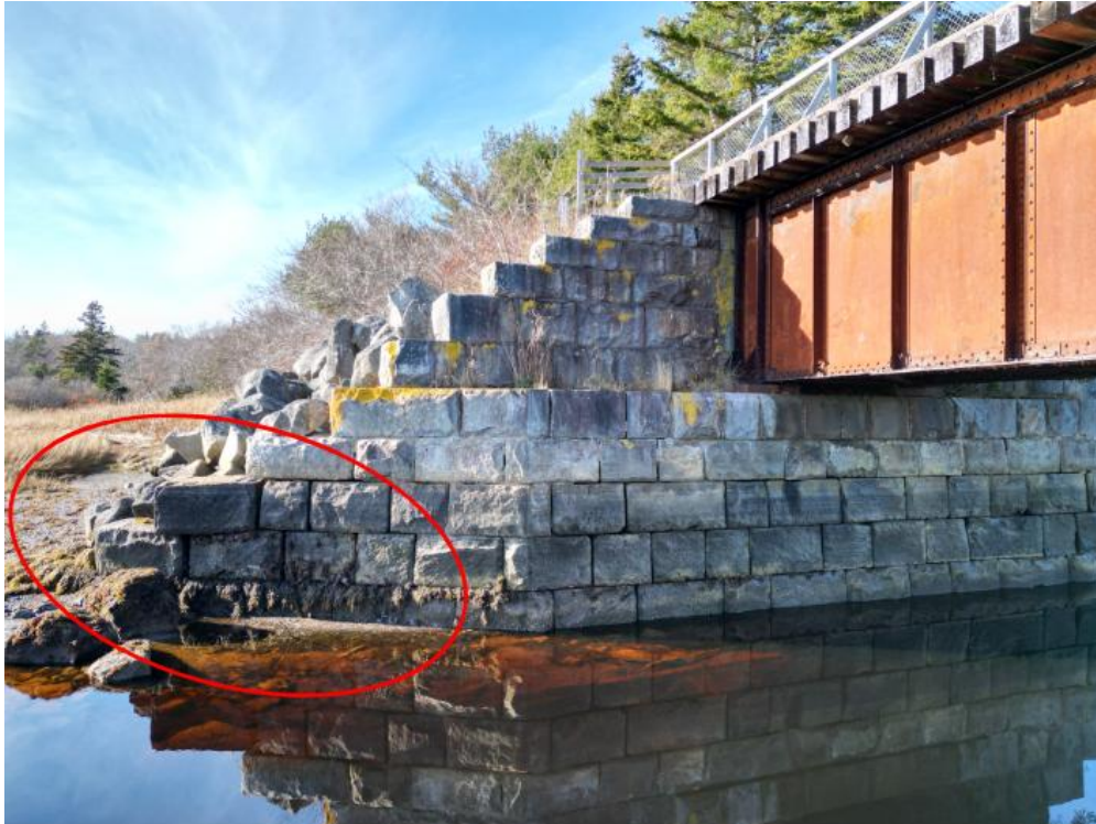
Photo 15: Dislodged masonry stones at the southwest abutment.
