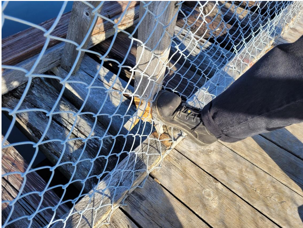
Photo 7: Typical view of a barrier post completely disconnected, north barrier.
