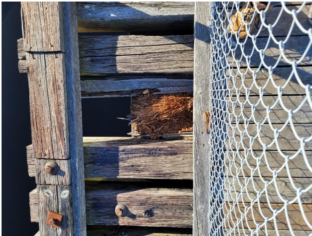
Photo 6: Typical view of a deteriorated timber tie, south side.
