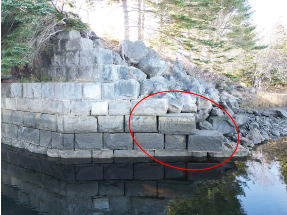
Photo 13: Dislodged masonry stones at the northwest abutment.
