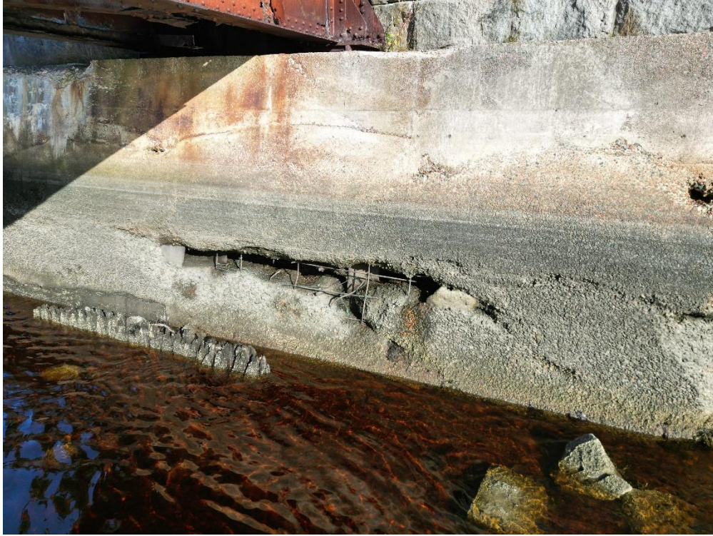
Photo 17: Severely eroded concrete jacket at the east abutment, with exposed reinforcement and other filler material (1).
