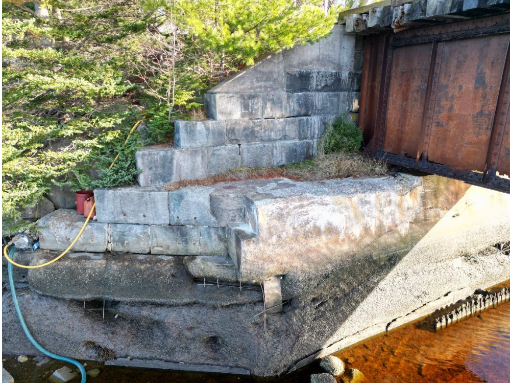
Photo 11: Cast-in-place concrete atop masonry stones at the east abutment near the girders.
