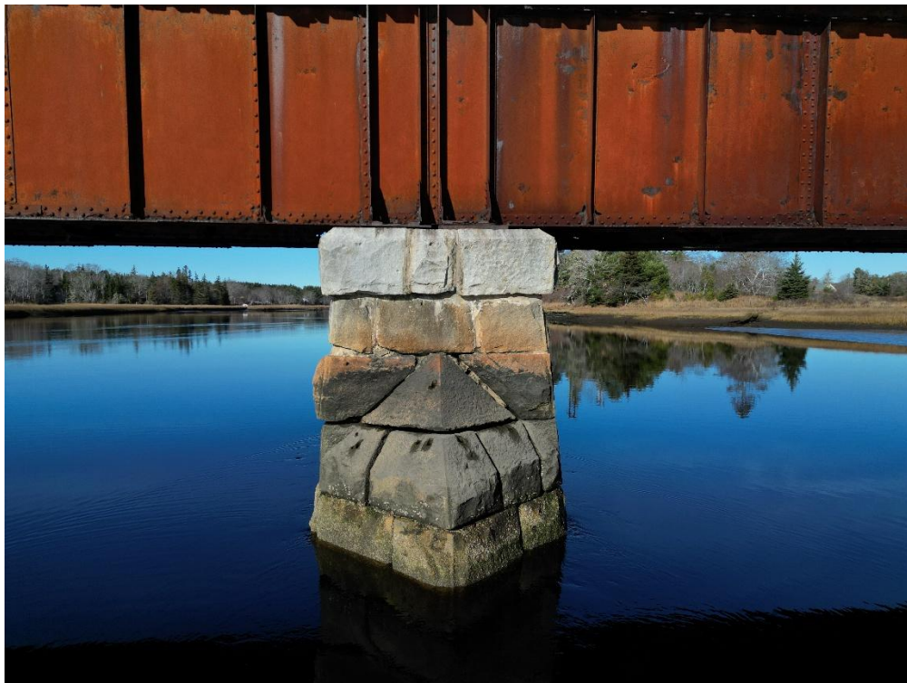
Photo 14: Slightly dislodged masonry stones on the south face of the piers.
