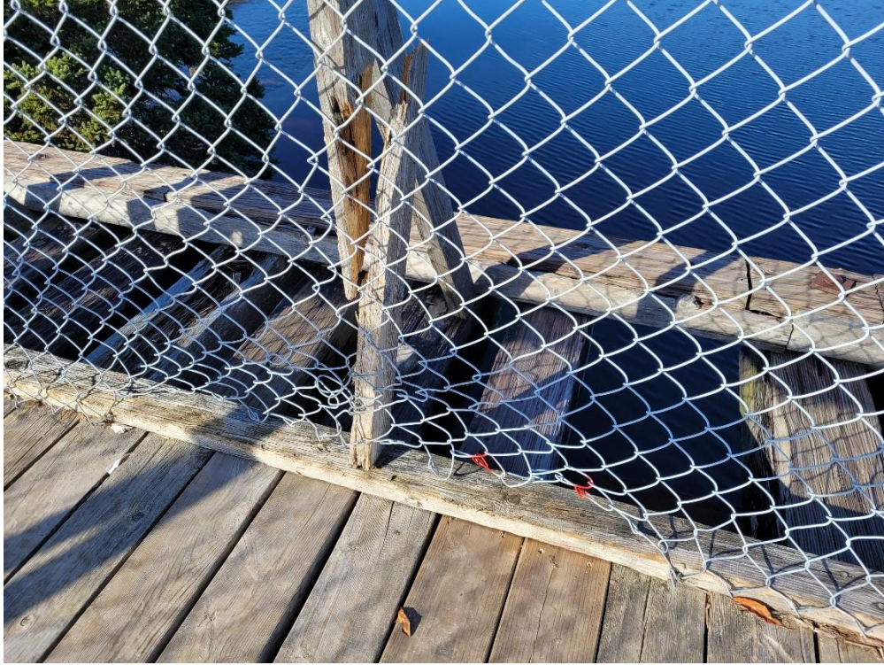
Photo 9: Barrier impact damage resulting in a damaged post, north barrier.
