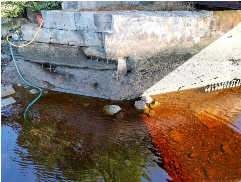
Photo 18: Severely eroded concrete jacket at the east abutment, with exposed reinforcement and other filler material (2).
