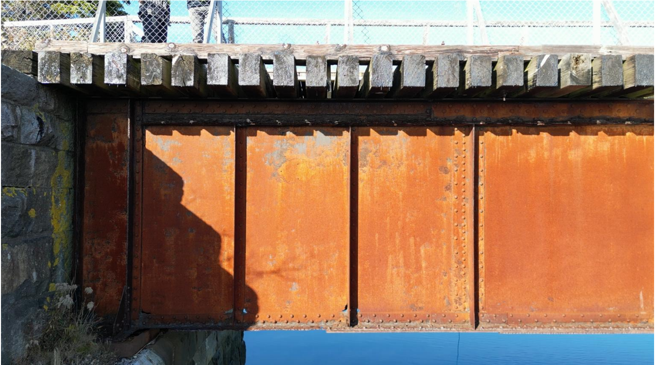
Photo 19: Severe corrosion on the south girder near the west abutment, resulting in section loss.
