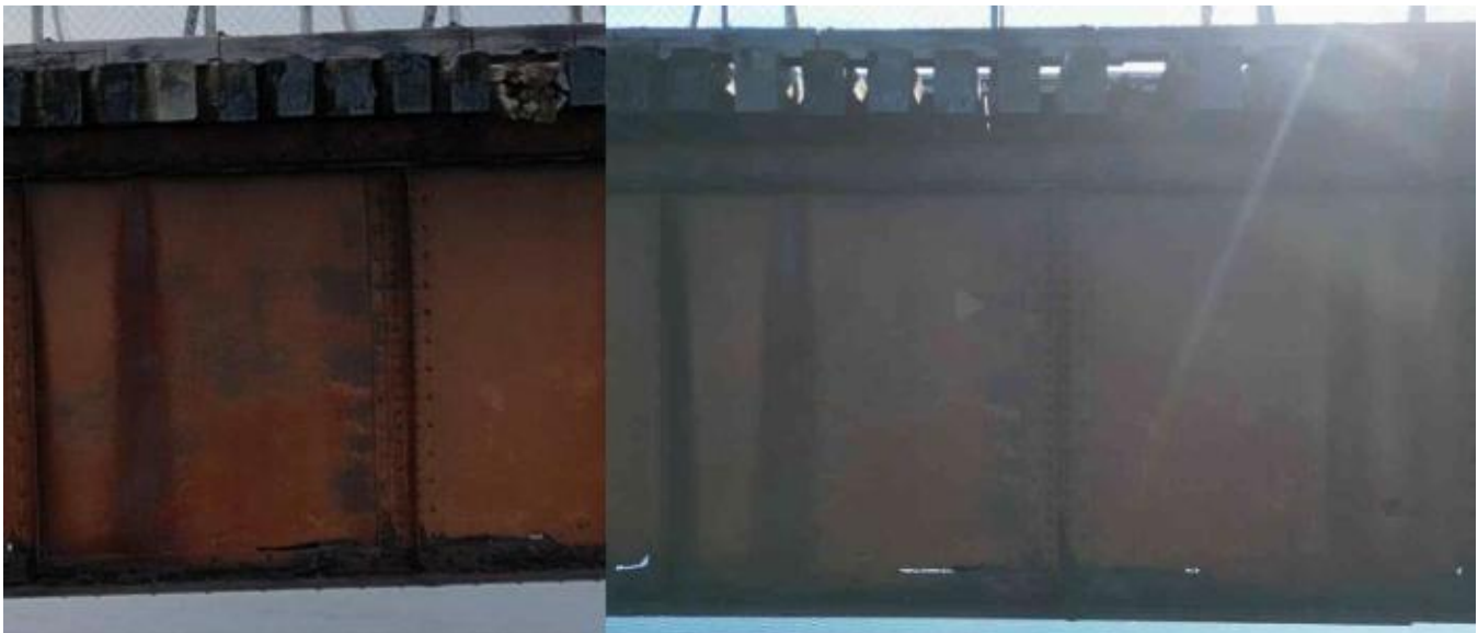
Figure 4 - North girder, Span 3 (viewed from west to east), showing condition comparison between 2023 (left) and 2025 (right). Similar conditions.
