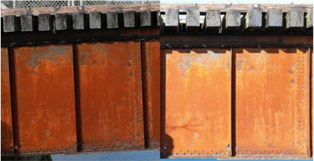
Figure 5 - South girder, Span 1 (viewed from west to east), showing condition comparison between 2023 (left) and 2025 (right). New section loss forming on the web and stiffener.
