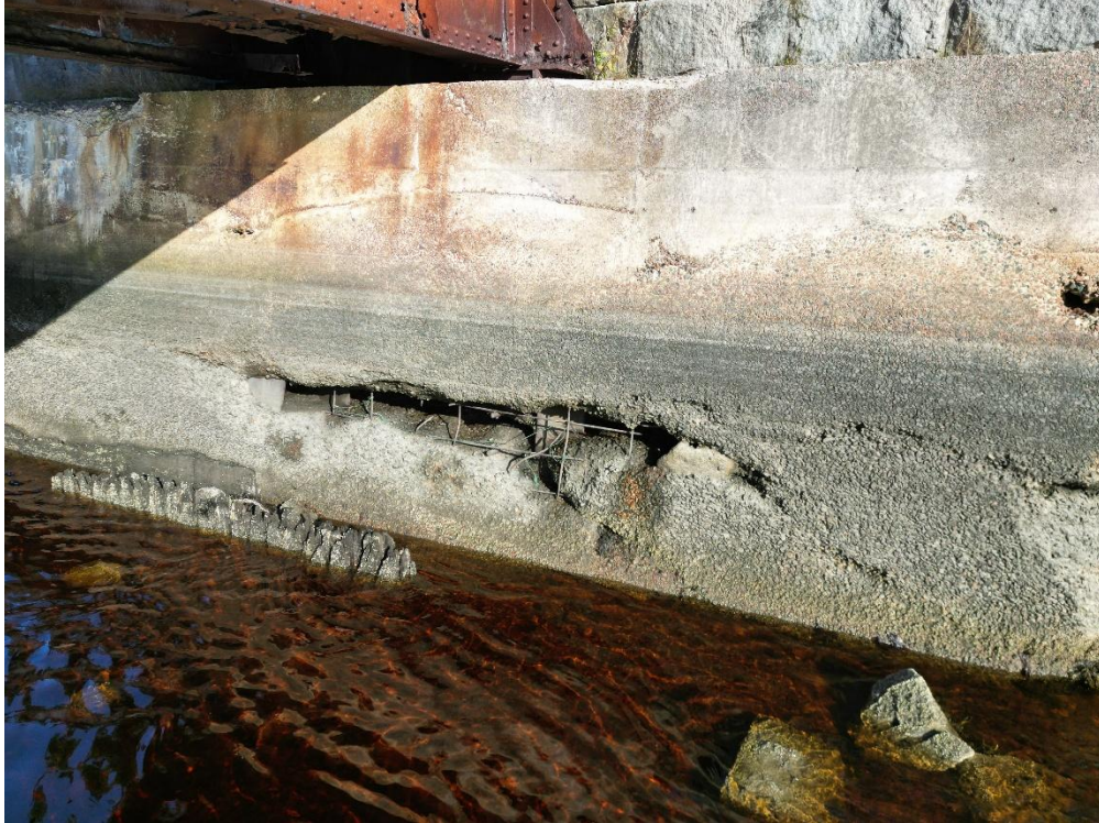
Photo 17: Severely eroded concrete jacket at the east abutment, with exposed reinforcement and other filler material (1).
