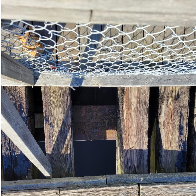
Photo 5: Typical view of a missing timber tie, south side.
