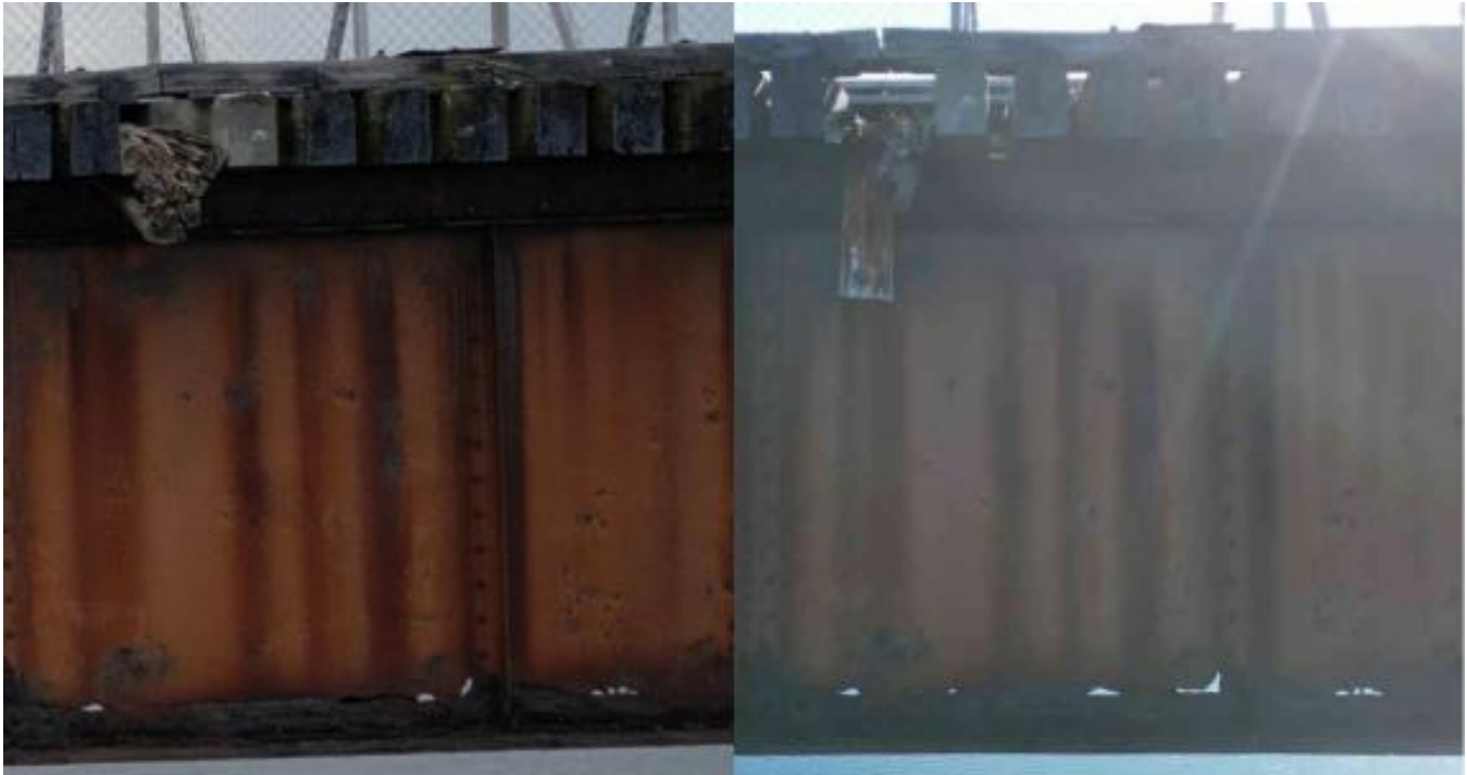
Figure 3 - North girder, Span 2 (viewed from west to east), showing condition comparison between 2023 (left) and 2025 (right). Increase in existing section loss and new areas of section loss forming.
