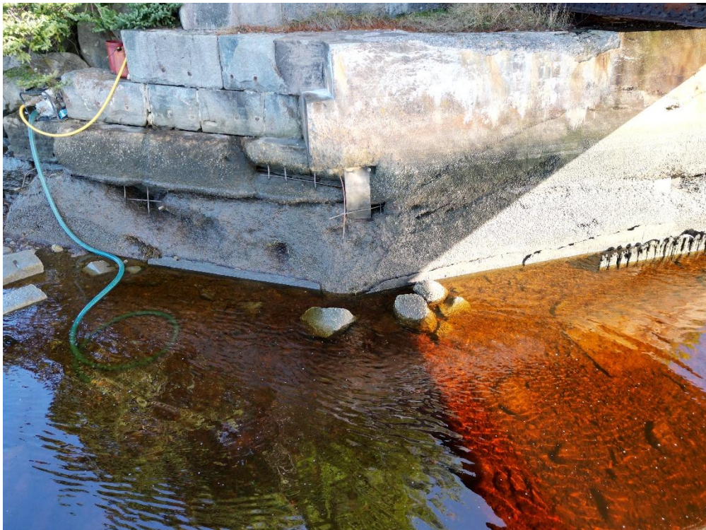
Photo 18: Severely eroded concrete jacket at the east abutment, with exposed reinforcement and other filler material (2).
