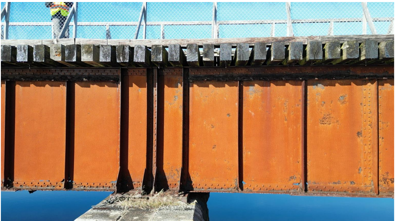
Photo 20: Severe corrosion on the south girder near the west pier, resulting in section loss.
