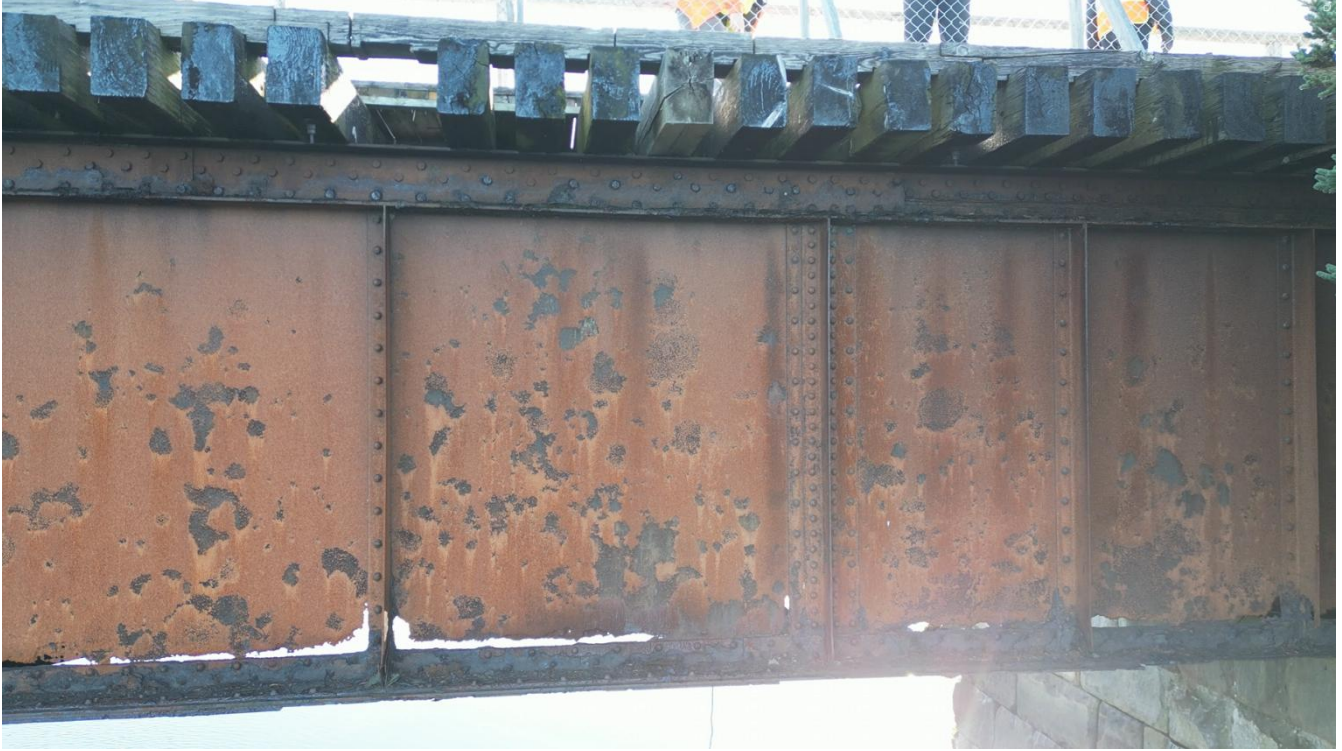
Photo 23: The most extensive corrosion on the north girder near the west abutment, resulting in severe section loss on the girder web.
