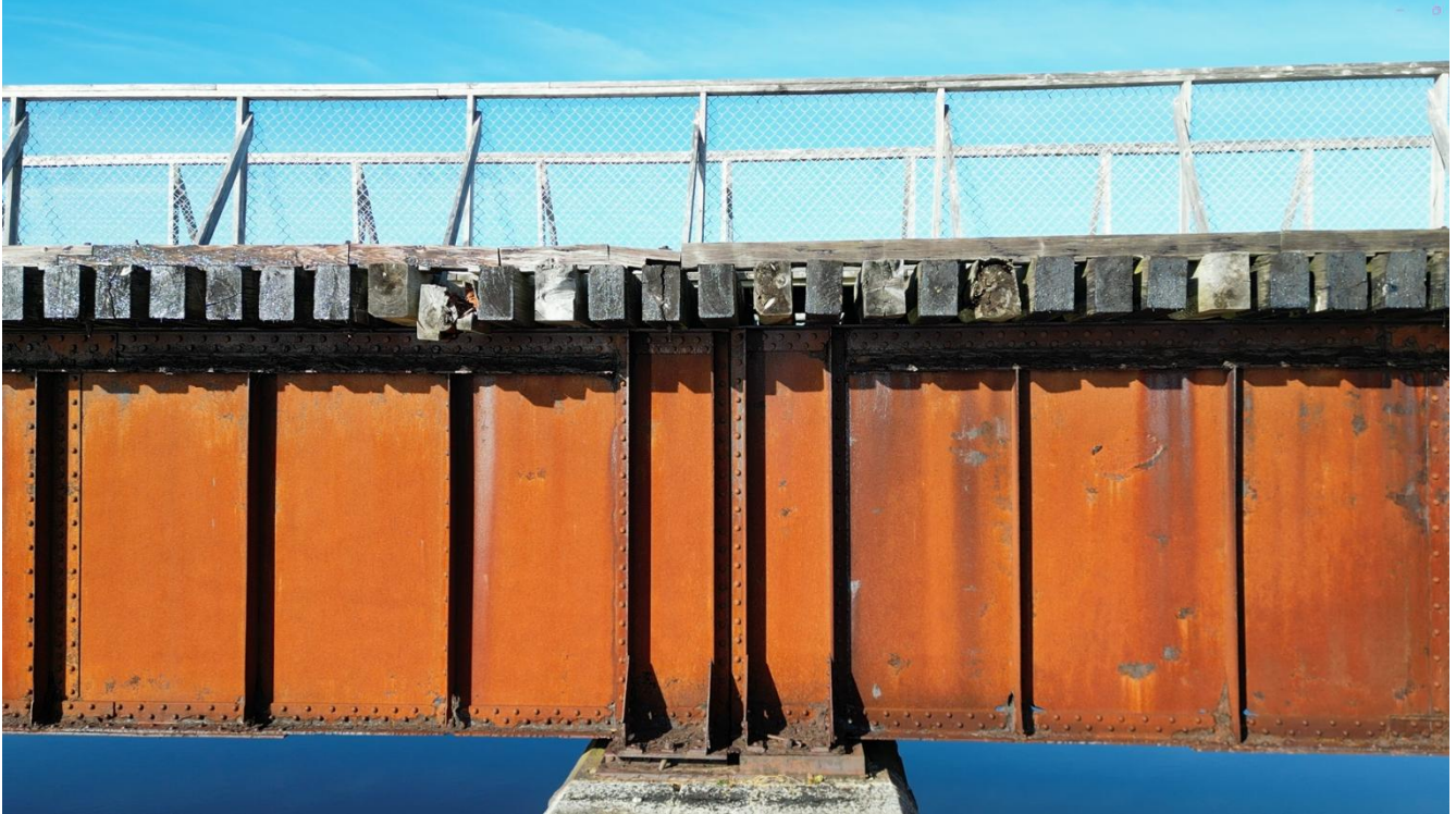
Photo 21: Severe corrosion on the south girder near the east abutment, resulting in section loss.
