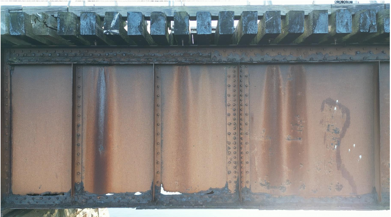
Photo 24: Severe corrosion on the north girder near the east abutment, resulting in section loss.
