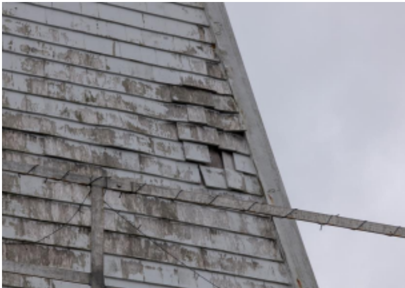
Figure 4: Damaged and missing wood shingles.
