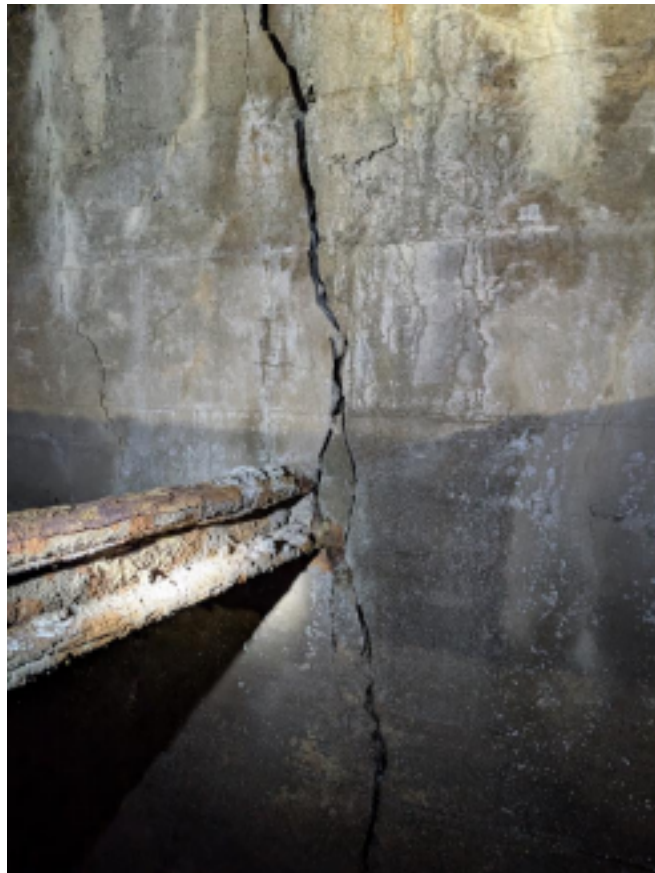
Figure 3: View of typical corrosion of steel bracing and large cracks in foundation wall.
