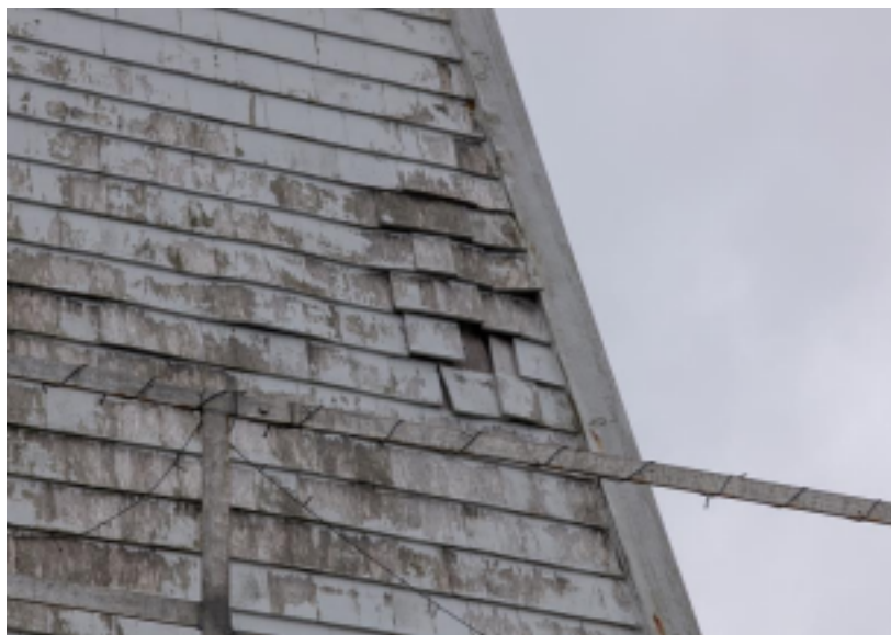
Figure 4: Damaged and missing wood shingles.
