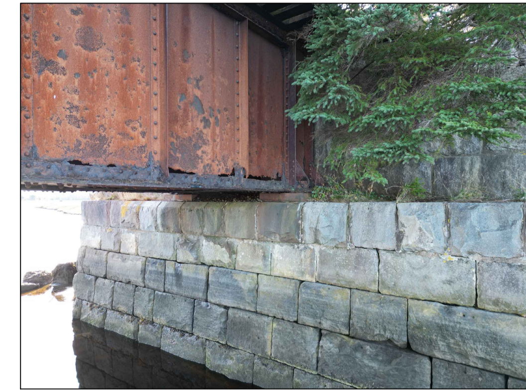
WEST ABUTMENT (MORTAR LOSS)
