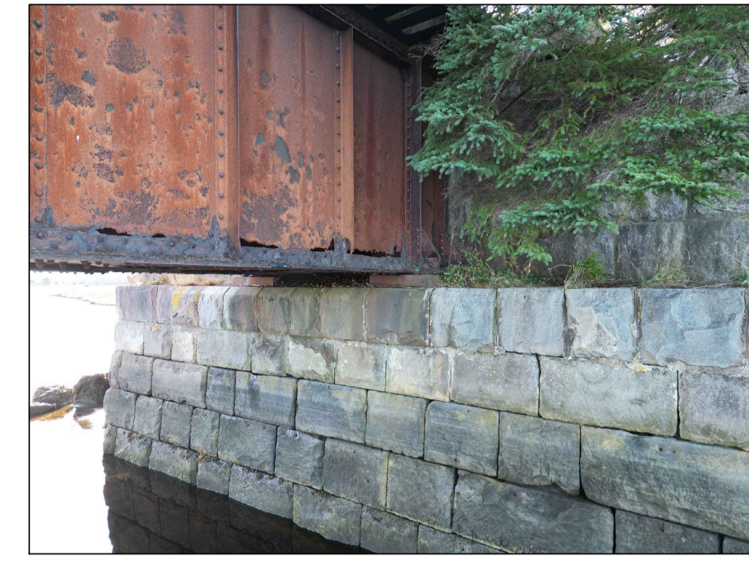
WEST ABUTMENT (MORTAR LOSS)
